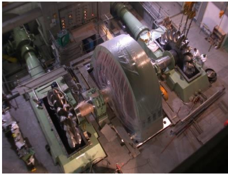
80 MW new generation Unit
