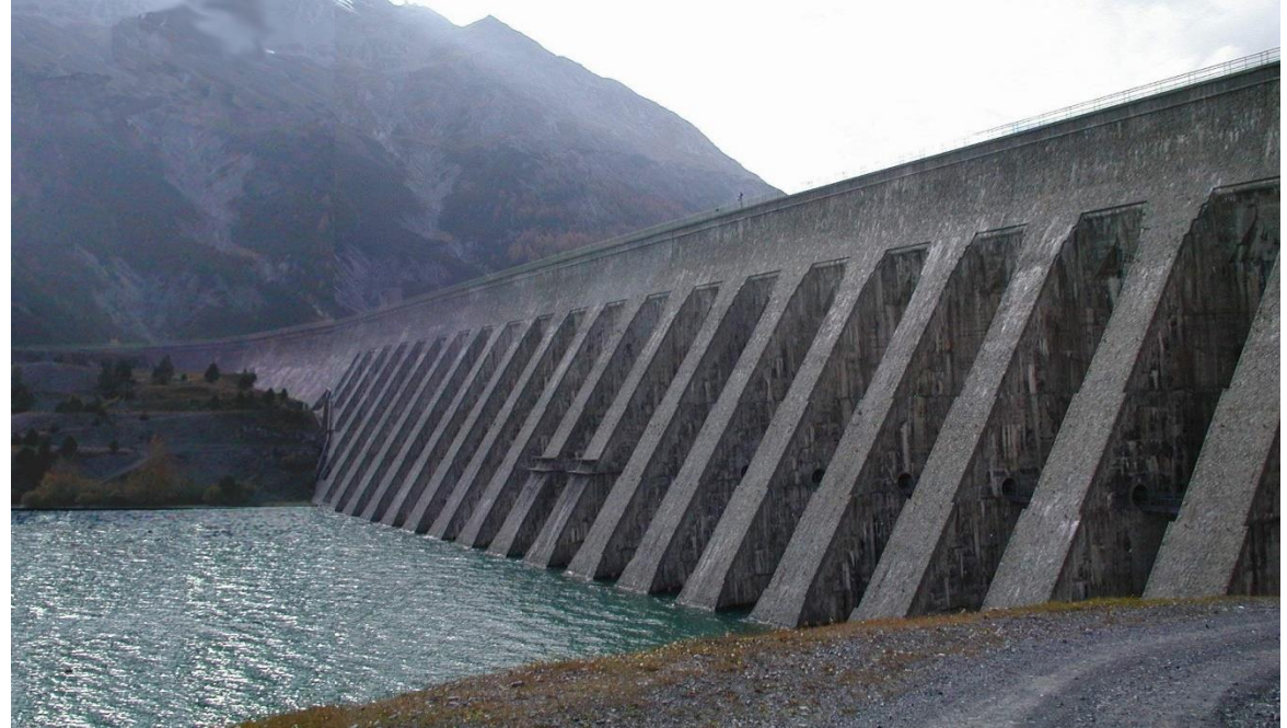
Old situation: water entering among the buttresses and therefore causing buoyancy of the barrage
