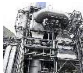
WTE Flue Gas Condensation system
